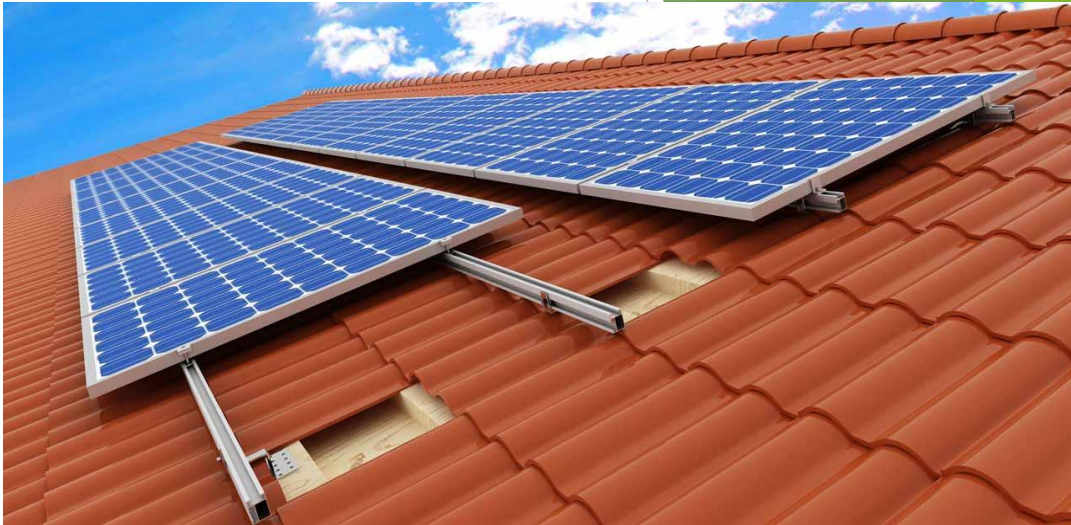
Image of roof mounted solar array
